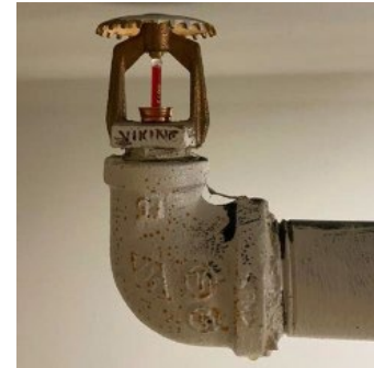
Close-Up of Sprinkler Head
